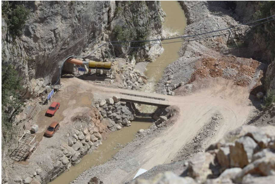
A construction site of the Ulog hydropower plant on the Neretva River, Bosnia and Herzegovina. © Robert Oroz
